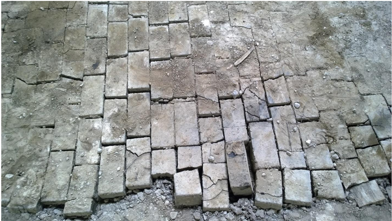
Evans Electric Building: Wood bricks absorbed the shock from pounding metal at the foundry.
