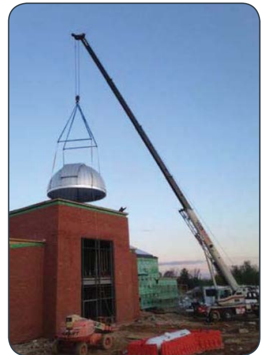
Dome being placed on top of the new APUS Information Technology Center
