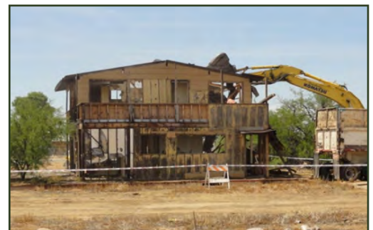
Properly demolishing buildings with asbestos containing material at the old feed lot brownfield site
