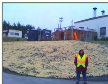
Interim Remedial Action at AOC D (Transformer Spill Site)
