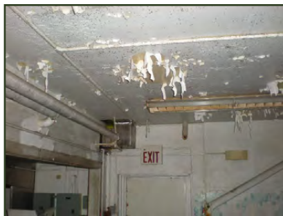
Abandoned school with flaking lead paint, mold and asbestos
