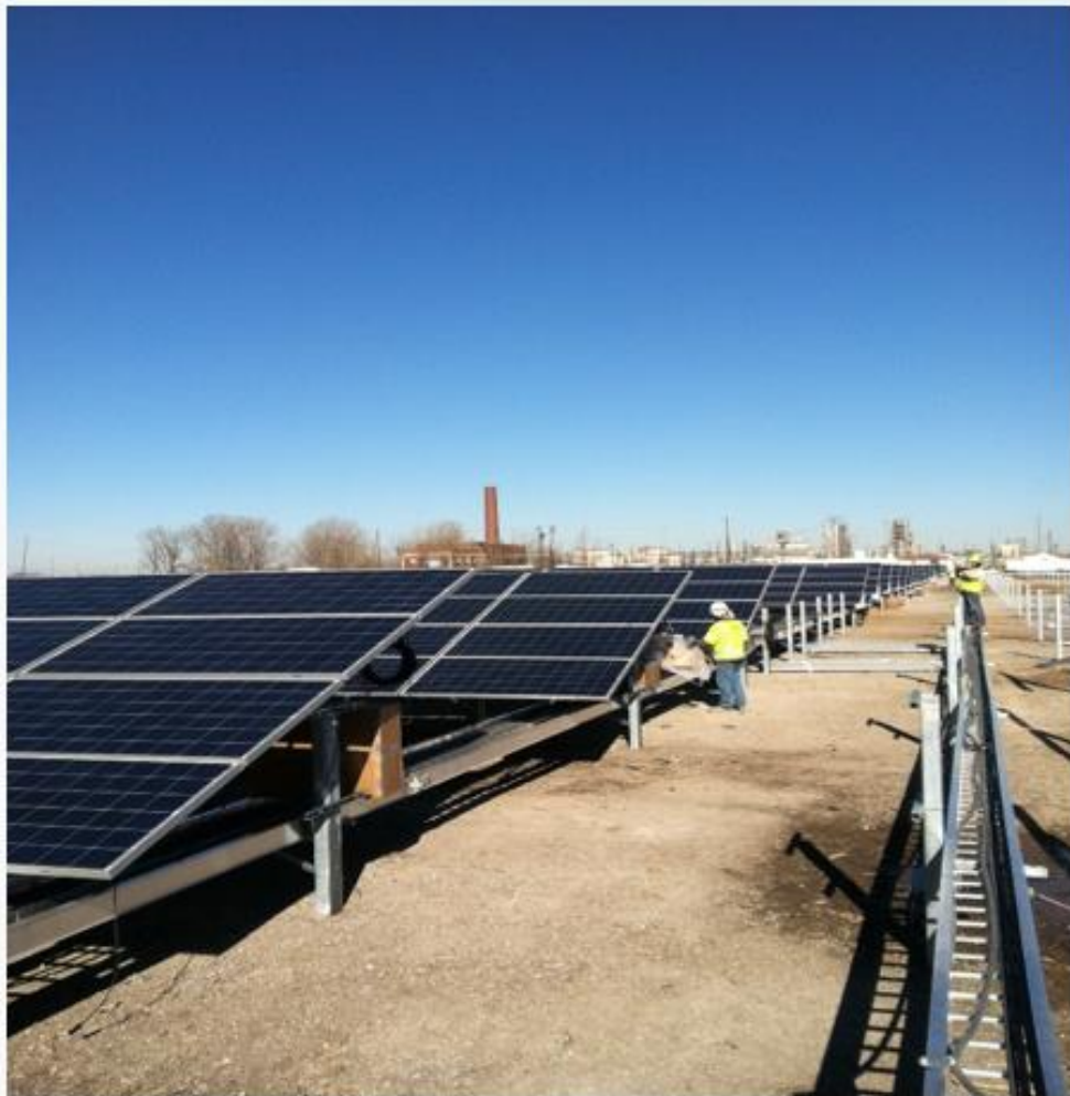
Construction of Maywood Solar Farm at former Reilly Tar & Chemical Superfund site, Indianapolis, Indiana
