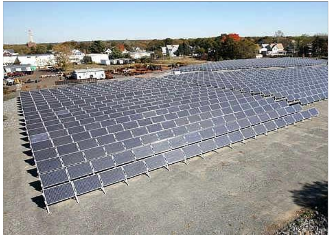
Brockton Brightfields, 425 kW solar PV
